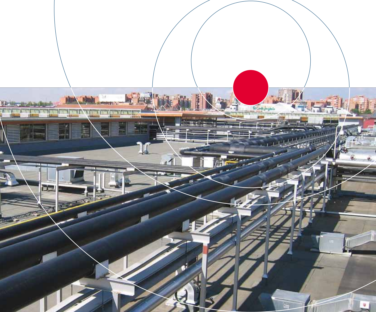
Cooling installation using LOGSTOR pre-insulated pipes (DN300–650) on the rooftop of the Parquesur supermall in Madrid, Spain in 2006.
